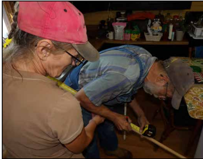
By Brent Engel, Public Relations Officer Linda and Jerry Lillard measure a parting stop for a window at their home. The couple participated in the USDA Rural Development Self-Help Housing program administered by NECAC.
