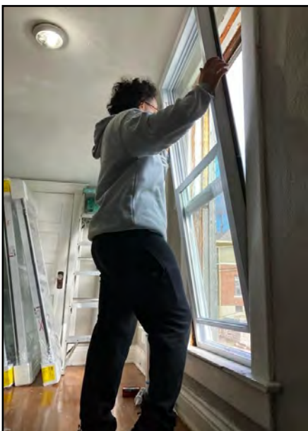
By Brent Engel, Public Relations Officer Roger Abbey installs a second-floor window at his Hannibal home.
